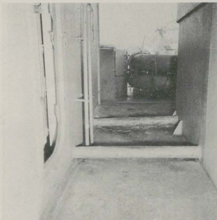
Photo 17: Looking to starboard through main deck passage-way at frame 91-1/2 showing wrinkles in deck plating. Four-inch pipe stiffeners were welded between deckhouses by ship's force.
