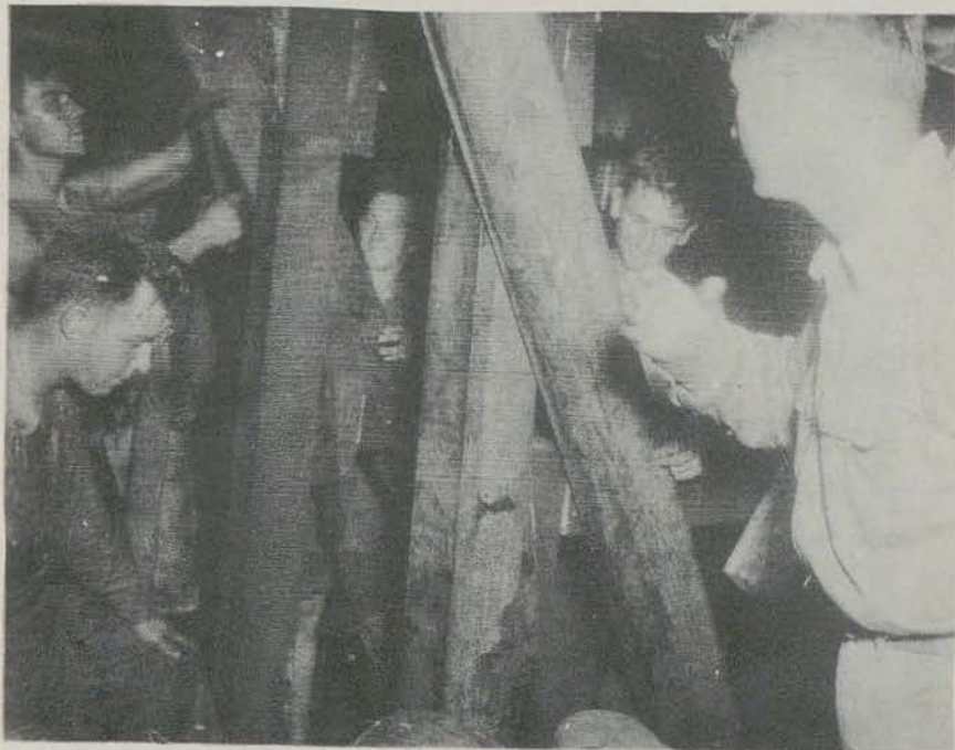
Photo 15: Shoring installed by ship's force against port side of bulkhead 88 in B-207-L.
